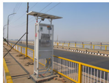
Remote water monitoring station in Allahabad (monitored parameters: TSS, COD, BOD, EC, pH, Temp, NH 4 , DO, Chloride, NO 3 -N)
