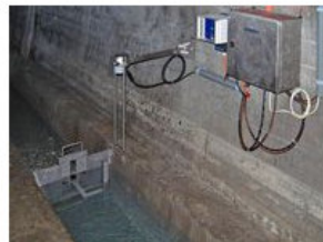
Automatic Leakage Water Measurement
